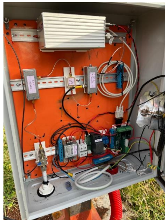
Figure 5: Complete electronics in enclosure
