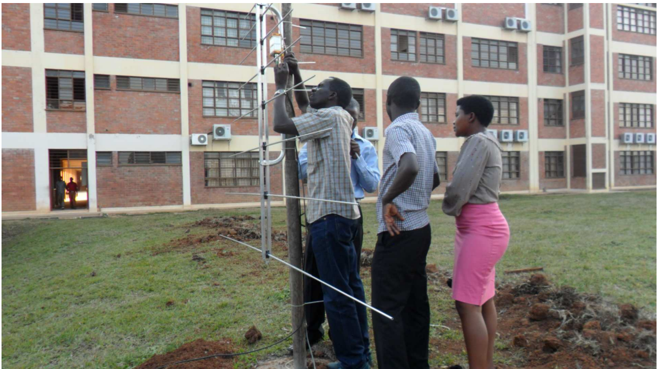
Figure 1 ~ Installation of a broad band logarithmic periodic dipole array (LPDA) and low noise amplifier (LNA) by students in the lawn in front of the college..
